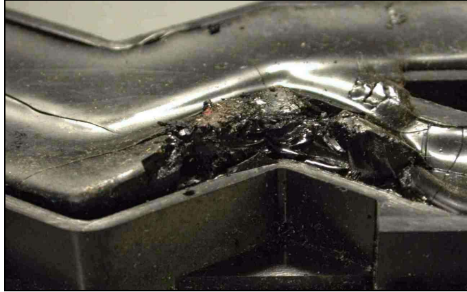
FIGURE 6 - OVERHEATING AT THE CONTACT BETWEEN THE BUSSBAR AND THE STAB SOCKET ASSEMBLY CAUSED THIS DAMAGE TO THE INSULATION. (This view is of the backside of the panel. The damage cannot be seen unless the panel is taken out of the enclosure.)
