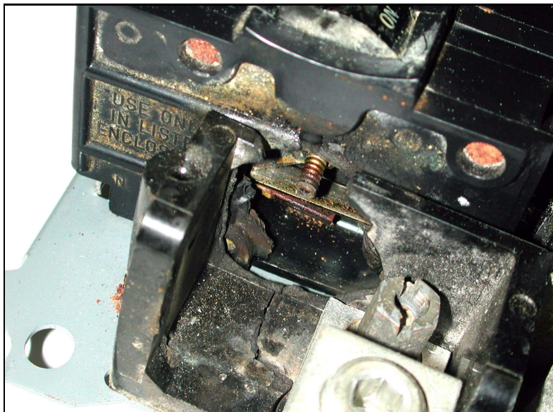
FIGURE 12 - VIEW DOWN TOWARD UPPER RIGHT OF PANEL SHOWN IN FIG. 11. THIS FPE STAB-LOK® TWO-POLE 30-AMP BREAKER FED THE CLOTHES DRYER.
