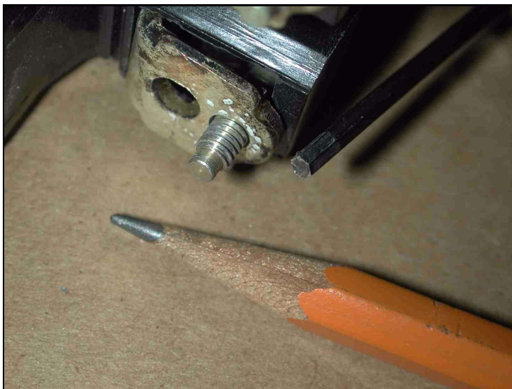
FIGURE 10 - ONE LOAD-SIDE CONTACT AND ITS 8-32 CLAMPING SCREW, ON THE FPE 100-AMP MAIN BREAKER OF FIG. 9. THE SCREW-HEAD TAKES A 3/32" ALLEN WRENCH, WHICH IS ONLY SLIGHTLY LARGER THAN THE LEAD OF THE PENCIL. (The larger hole next to the clamping screw provides clearance for the end of the screw that protrudes from the mating contact plate)
